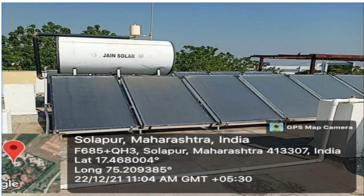
Rooftop Solar Panels
